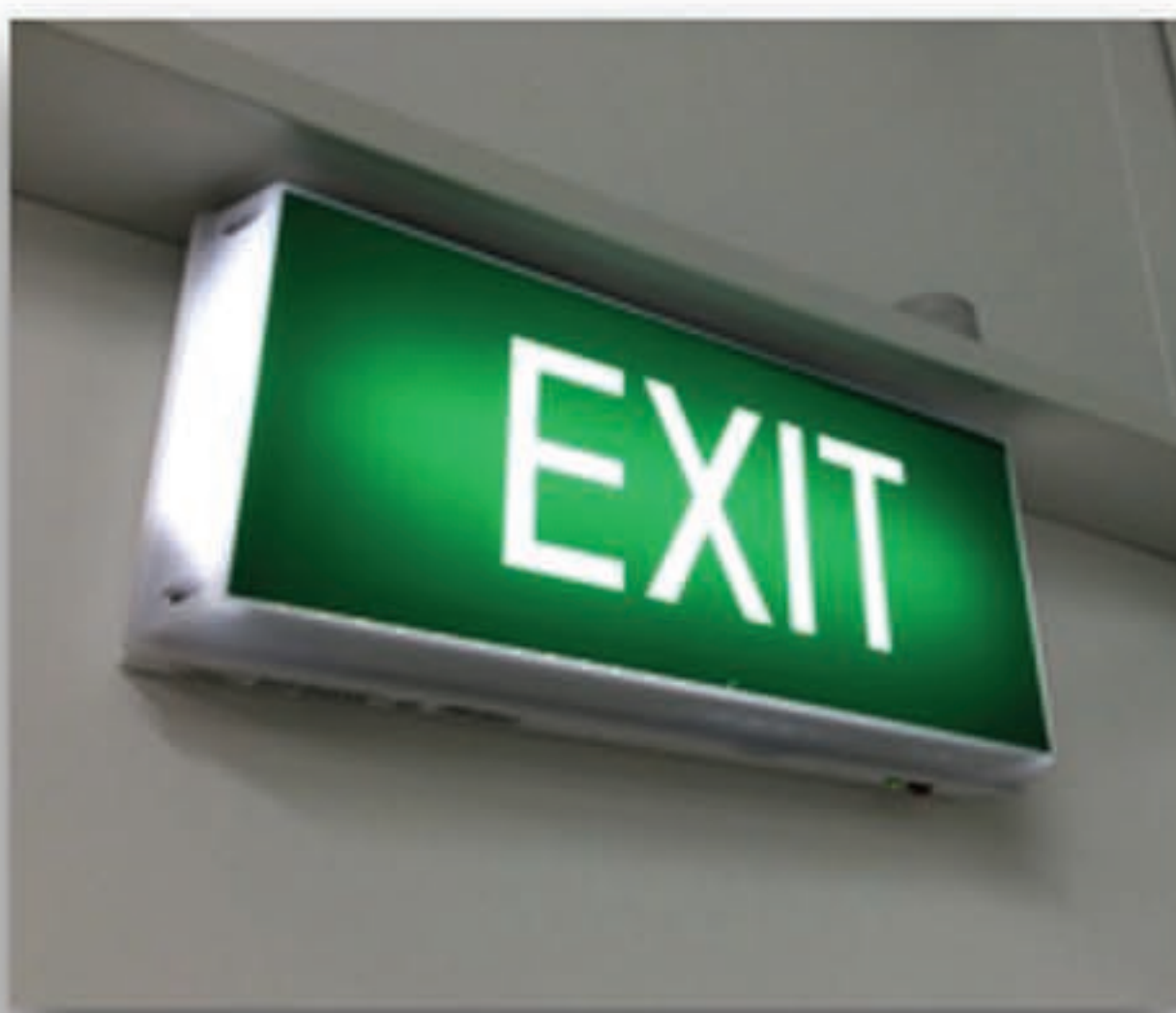
EXIT sign lamp
